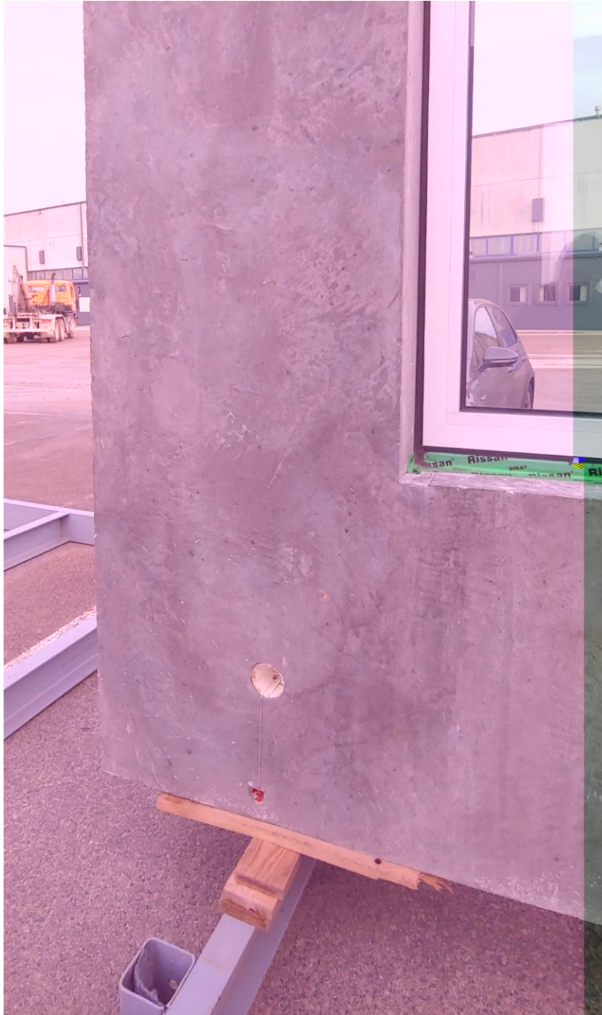
ELECTRICAL OUTLET in BASE PANEL
