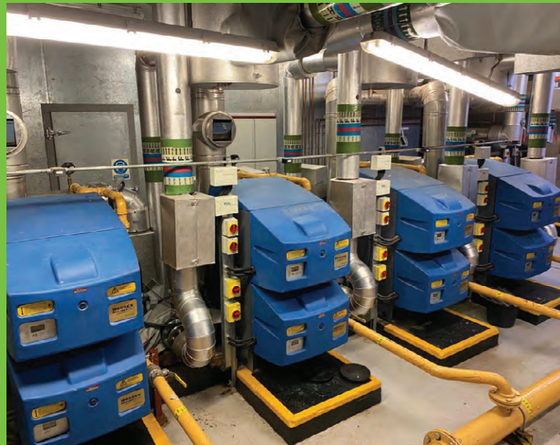
Boiler plant room at one of the bank's EndoTherm installations.
