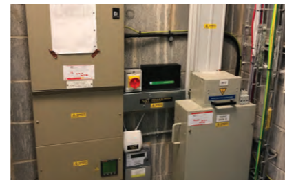
MKL's installation (shown as the black box) at Mott McDonald.
